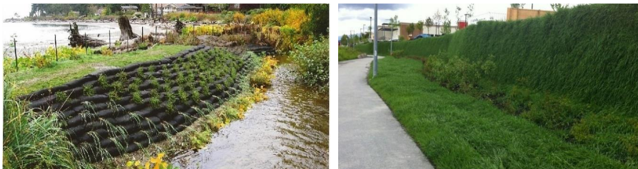
Image 5.8: Example of steepened slope reinforced soil embankment (left before growth, right after growth)
